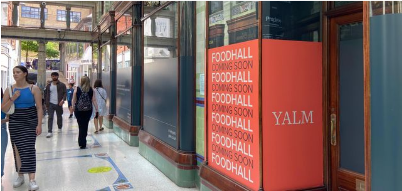
Works to ready the food hall began in July - Credit: Maya Derrick
