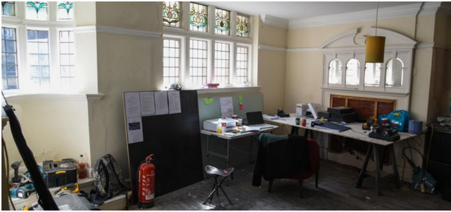
The private dining area at Yalm - currently being used as a site office while building work is under way - Credit: Danielle Booden
