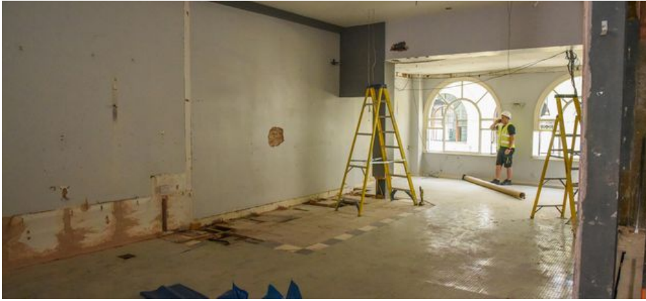
Kitchens will be fitted in this space off the main dining hall - Credit: Danielle Booden
